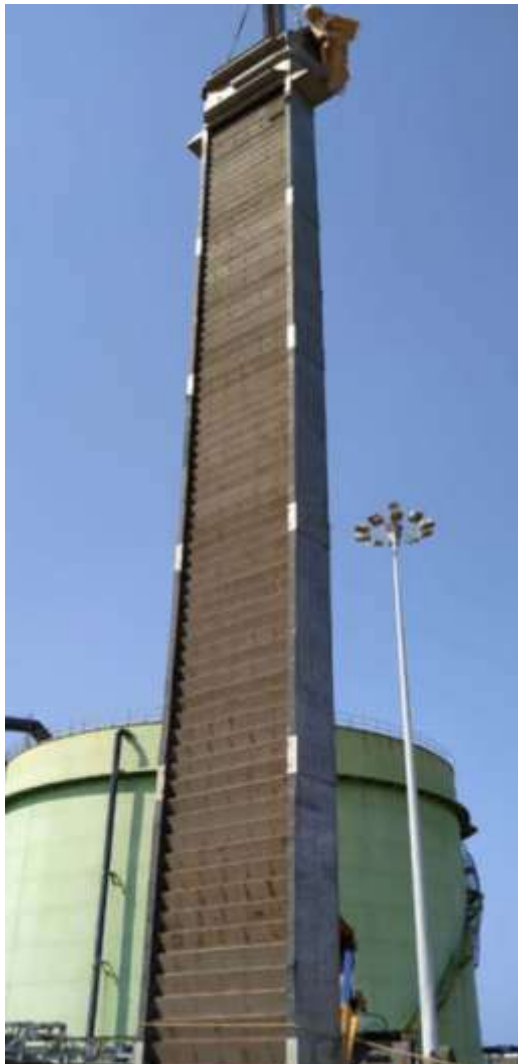
Screen having 18 m length during installation at Nemmeli Desalination Plant, Chennai (India)
