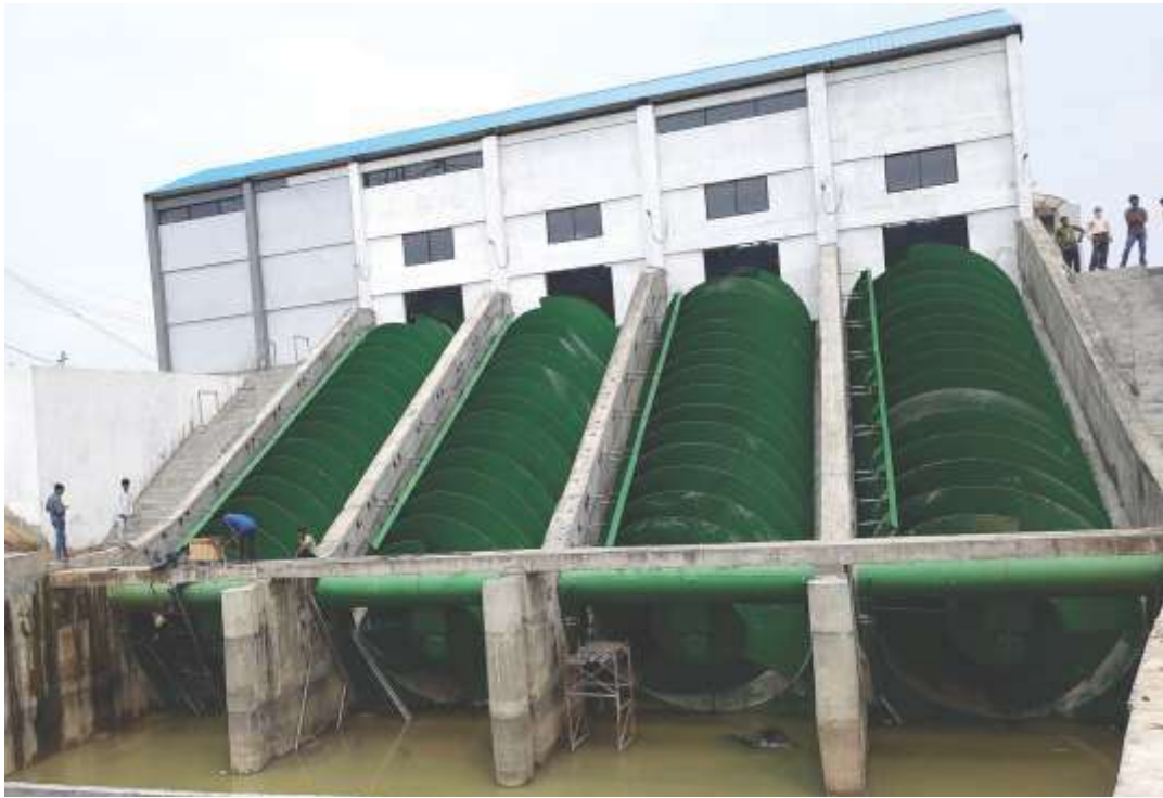
Hydro Screw Generator SSNNL Project, Gujarat
