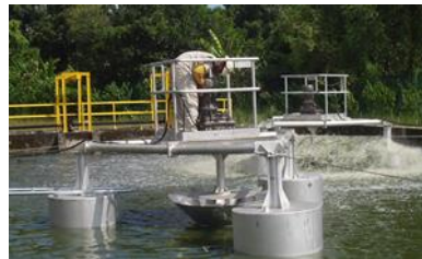
Slow speed floating aerator
