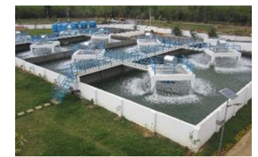
Slow speed fixed aerator
