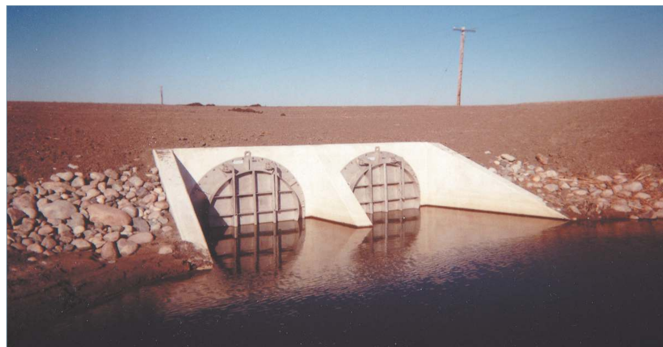
Two 1500 mm Diameter Flap Gates help protect a North Dakota watershed from forward and reverse surges.
