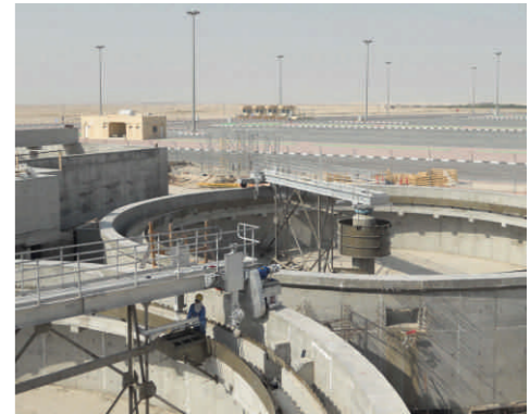
Stainless Steel Clarifiers at STP, Doha, Qatar
