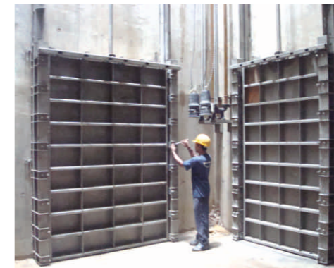
SS Sluice Gates at Punggol Serangoon Water Pumping Station, Singapore.
