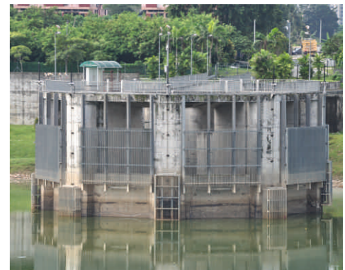
Sluice Gate & Trash Screen at Kerajaan Storm Water Management and Road Tunnel Project, Kuala Lumpur, Malaysia
