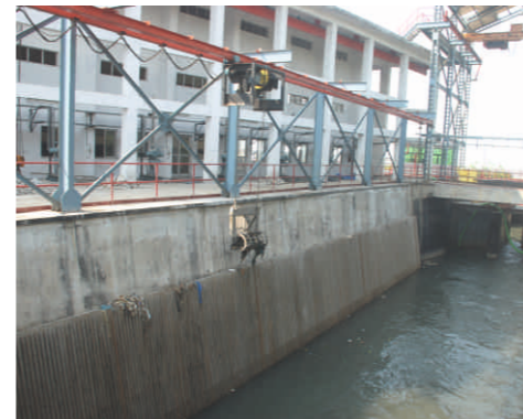
Suspended Trash Rake Screen and Sluice Gate at Haji Ali Storm Water Pumping Station, Mumbai, India
