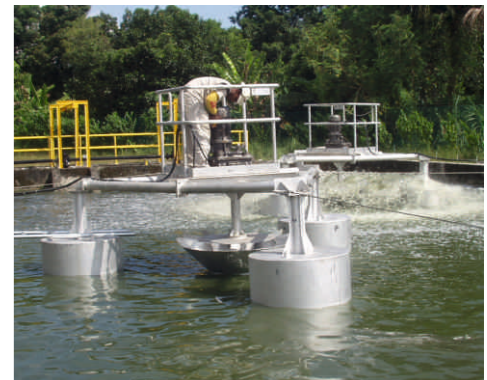
Floating Surface Aerators installed at Sewage Treatment Plant, Ipoh, Malaysia.
