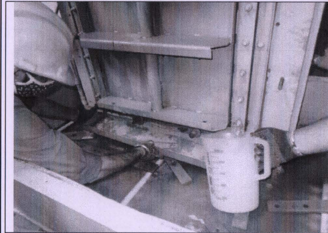
Description: Observed leakage rate after complete 100000 cycles (Found 220ml).
