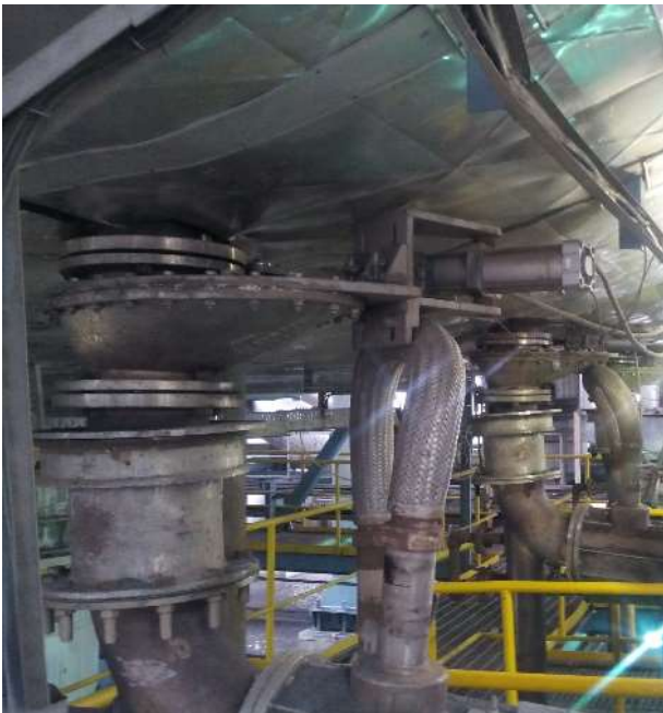
KU-HT DN200 Installed at M/s Bajaj Energy Ltd.
