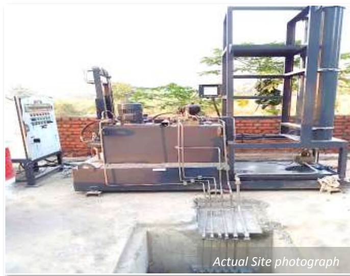
Under testing at plant
