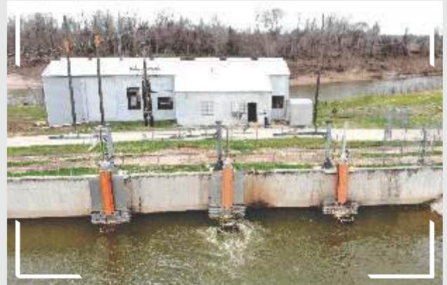
GCWA Pump House Levee Structure, Sienna Parkway, TX, USA Knife Gate Valve Dia. 72" - 3 nos.
