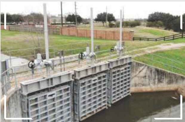
GCWA, Sienna Parkway, TX, USA CI Sluice Gate 8' x 8' - 3 nos.
