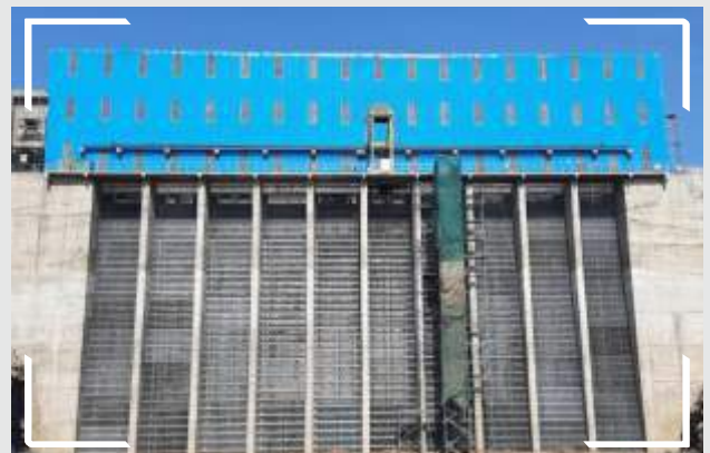
Kundalia Lift Irrigation Package, M.P. India Trash Rack Grab Cleaner Mechanism 31 m height and 4.5 m width ( Per bay width). Total no of bay is 10 - 3 nos.
