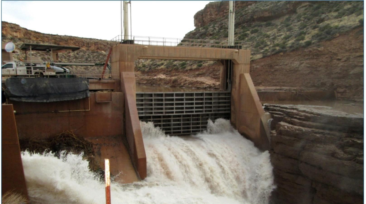
480" x 240" Stainless Steel Roller Gate for Quail Creek Reservoir, UT, USA Comprised of two 480" x 120" Gates, Operating Independently to Provide Overflow or Aperture Discharge
